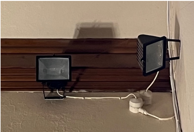
Photo 26 – Flood Lights in the South Transept
