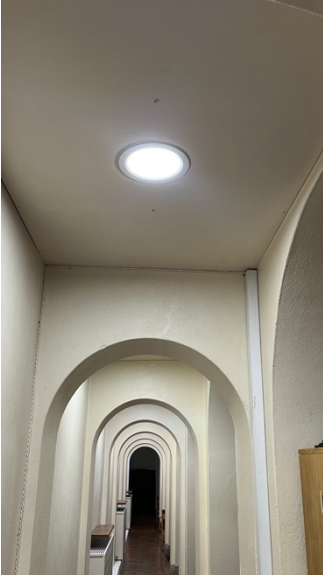
Photo 22 – Colonnade ceiling lights
